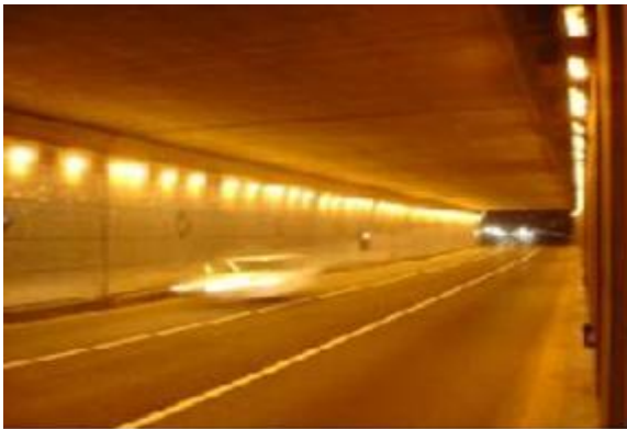
Before: 250W High Pressure Sodium
