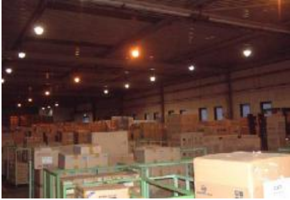
Before: 175W HPS and 150W Metal Halide
