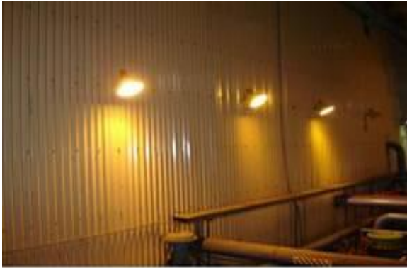
Before: 175W High Pressure Sodium
