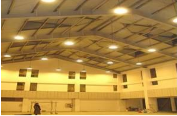
Before: 400W High Pressure Sodium
